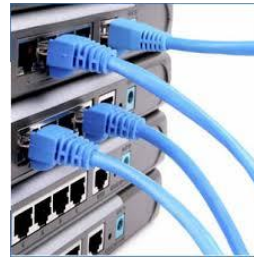
Network Installation & Support Services
